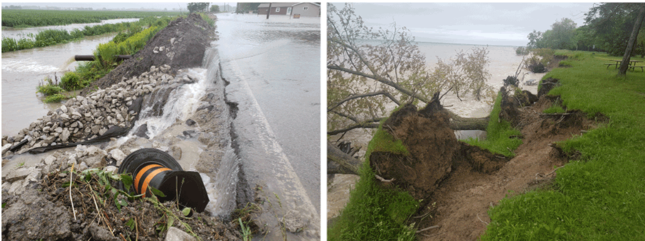
Figure 3.11: Left: Eroding bluffs along Lake Erie at Wheatley Provincial Park in 2018. Right: August 27, 2019 flooding at Erie Shore Drive. Increased shoreline erosion and flood risk are attributed to changes in lake levels, ice cover and exposure to wave energy. Source: Zuzek, 2020.
